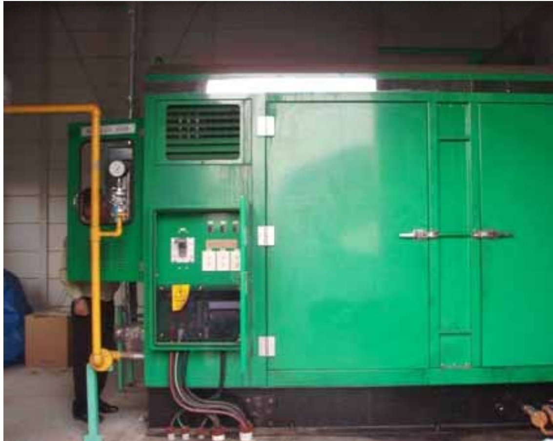
Generator(Dual fuel type)
