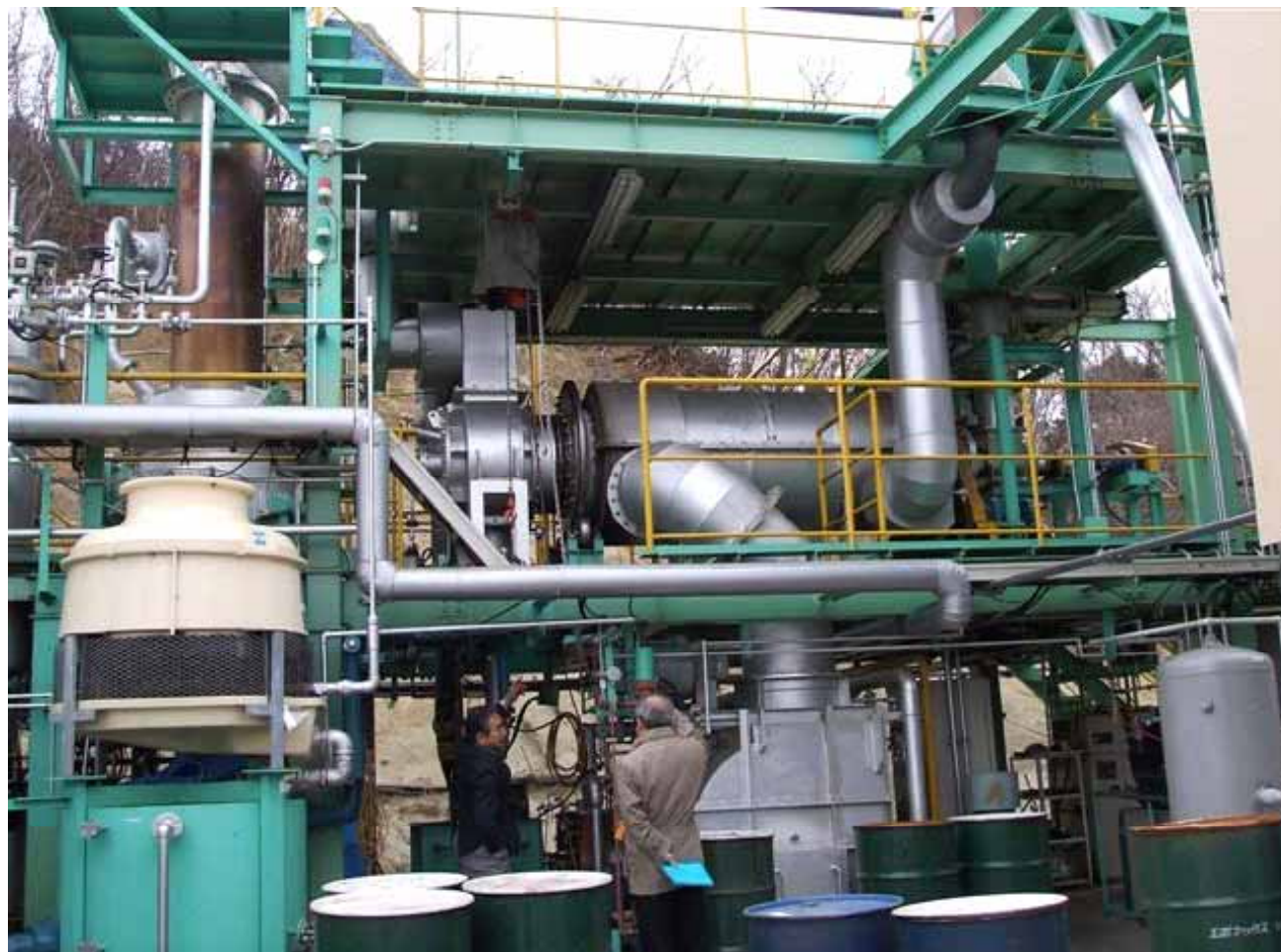
Photo 1 Gasification Plant in Iwaki City
